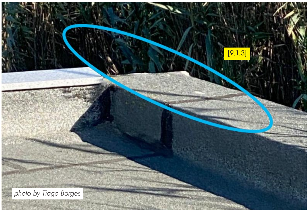
9.1.3. Lack of capping on the wall on the east side, roofing felt not properly welded.
