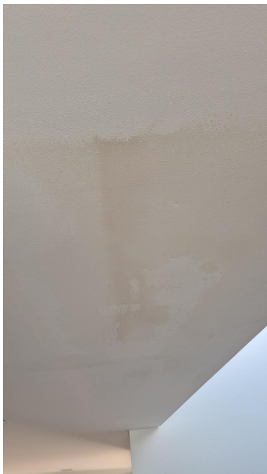
Stains on the corridor ceiling.
