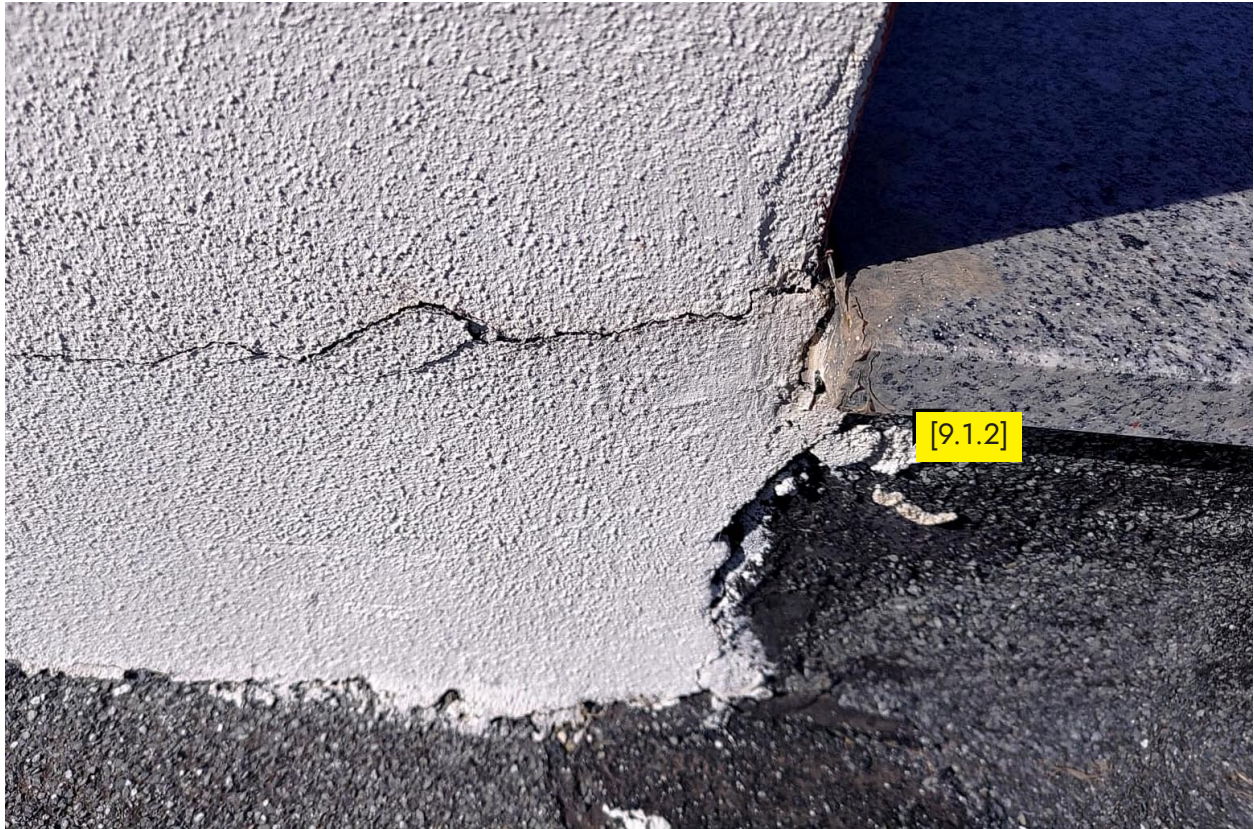
9.1.2. Cracks at the connection of the attic to the walls of the pergola and the house.
