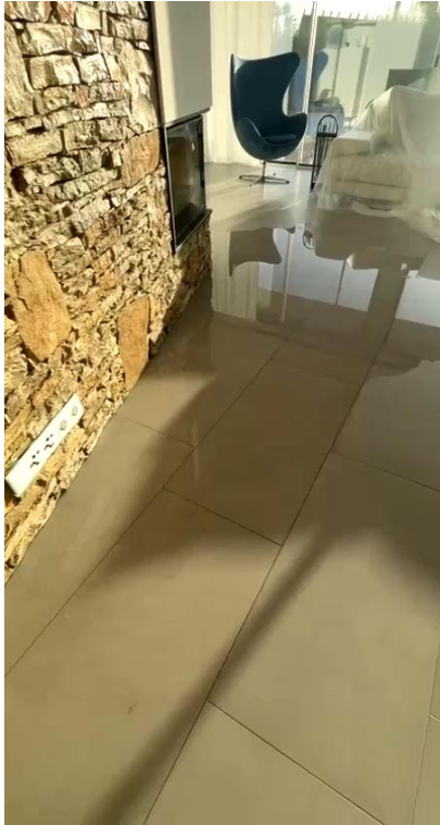
Rainwater flooding on January 2025
