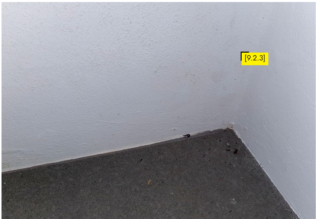
9.2.3. Crumbling plaster, soggy paint coming off.
