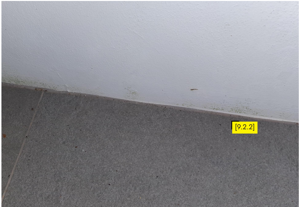
9.2.2. Damp patches on the walls. Green algae growth in plaster.
